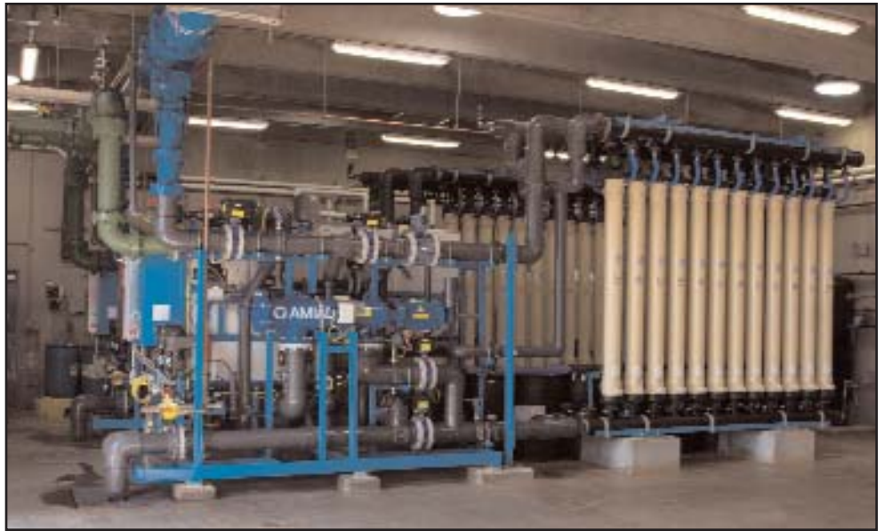
The heart of the Bealeton microfilter plant is the system of pumps and large filters, through which the water from all three wells is cleaned. Photo courtesy of Emery and Garrett Groundwater Investigations Inc.
