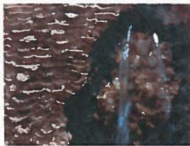
Groundwater Leaking into Sewer
